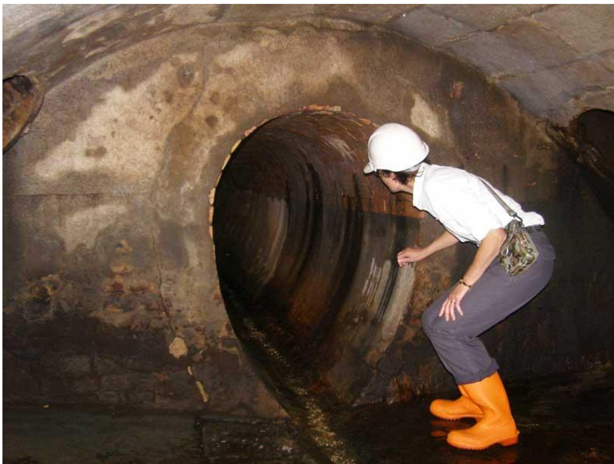
Figure 2.5: Section of brick oviform drain joining arched stone section of Tank Stream. Google
