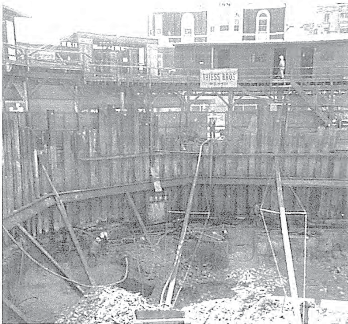
Figure 3.15: 1965 image showing the excavation and shoring for the below-ground levels of the Gold Fields House development. This view is looking east to Pitt Street, note the bystander on street level (beneath the Theiss sign). The tank stream is in Pitt Street behind the shoring. (Source: City of Sydney Council Archives)
